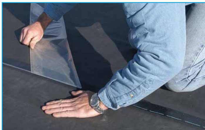
Seams completed with Versico's QAT Seam Technology go together smoothly, resulting in fewer wrinkles.
